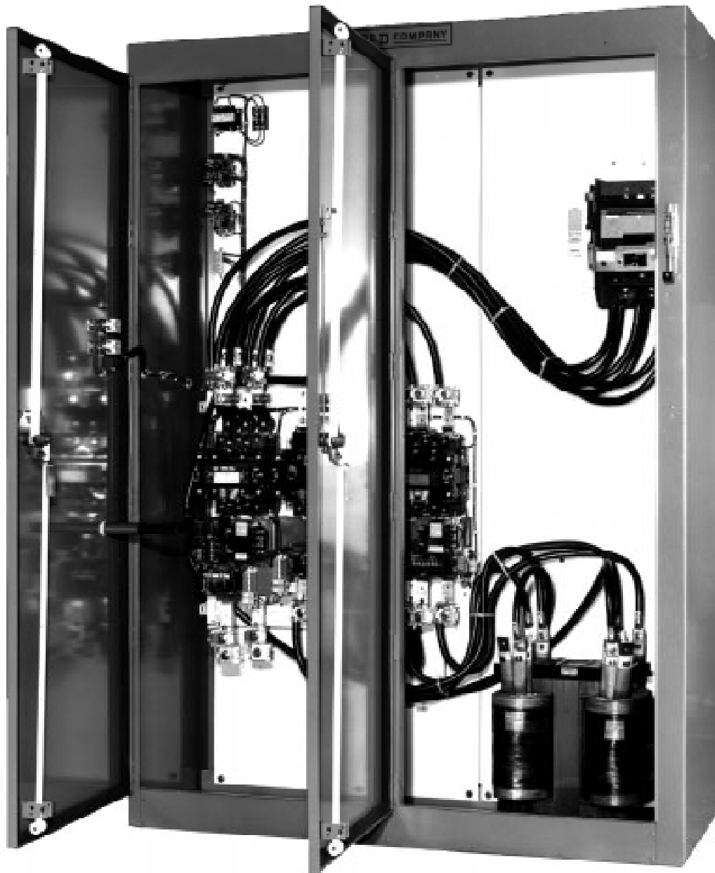
Figure 3 Class 8606 Type SJA11UV81 Forms A FF4TY791 Size 7 Size 7 Autotransformer Starter in NEMA 12 enclosure with circuit breaker and 120 VAC CPT for timing relay and START/STOP push buttons for 600 hp / 480 VAC motor.
