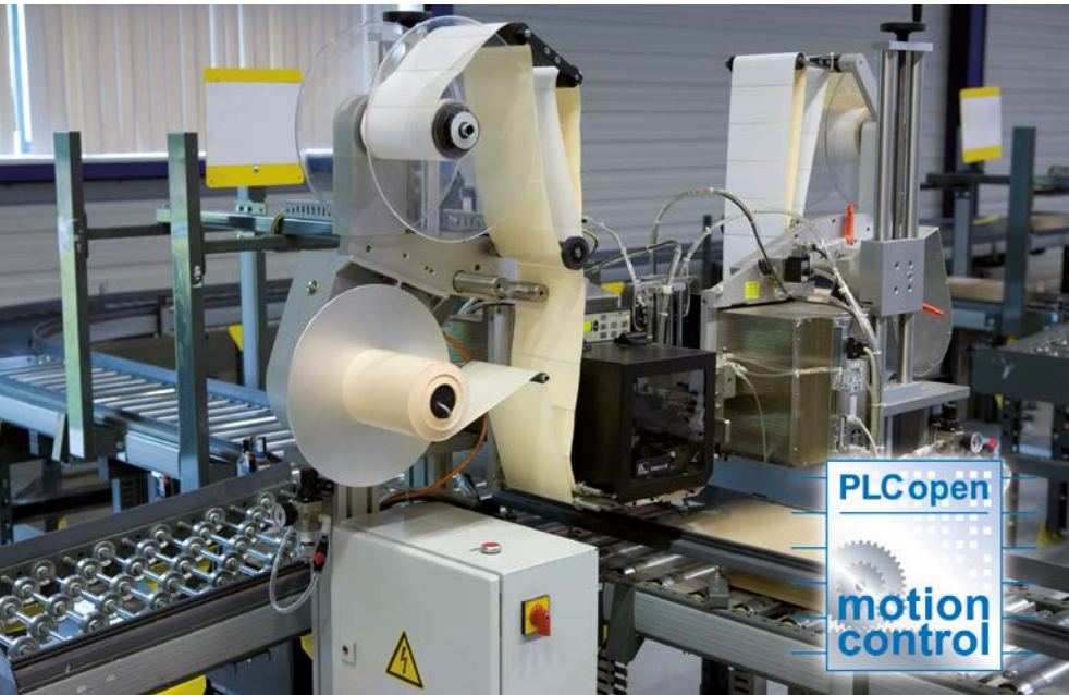
Labelling machine controlled by a L series PLC in combination with a Simple Motion module.
