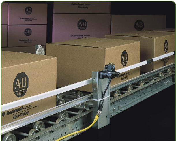
Material handling application – A retroreflective RightSight detecting packages on a conveyor line.
