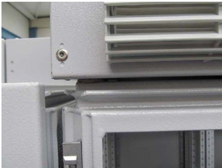
Figure 3-19 View with opened cabinet door
