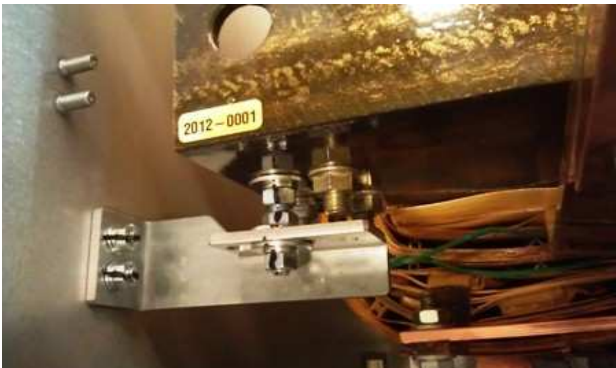
Figure 6-5 Transformer fixing on the left side
