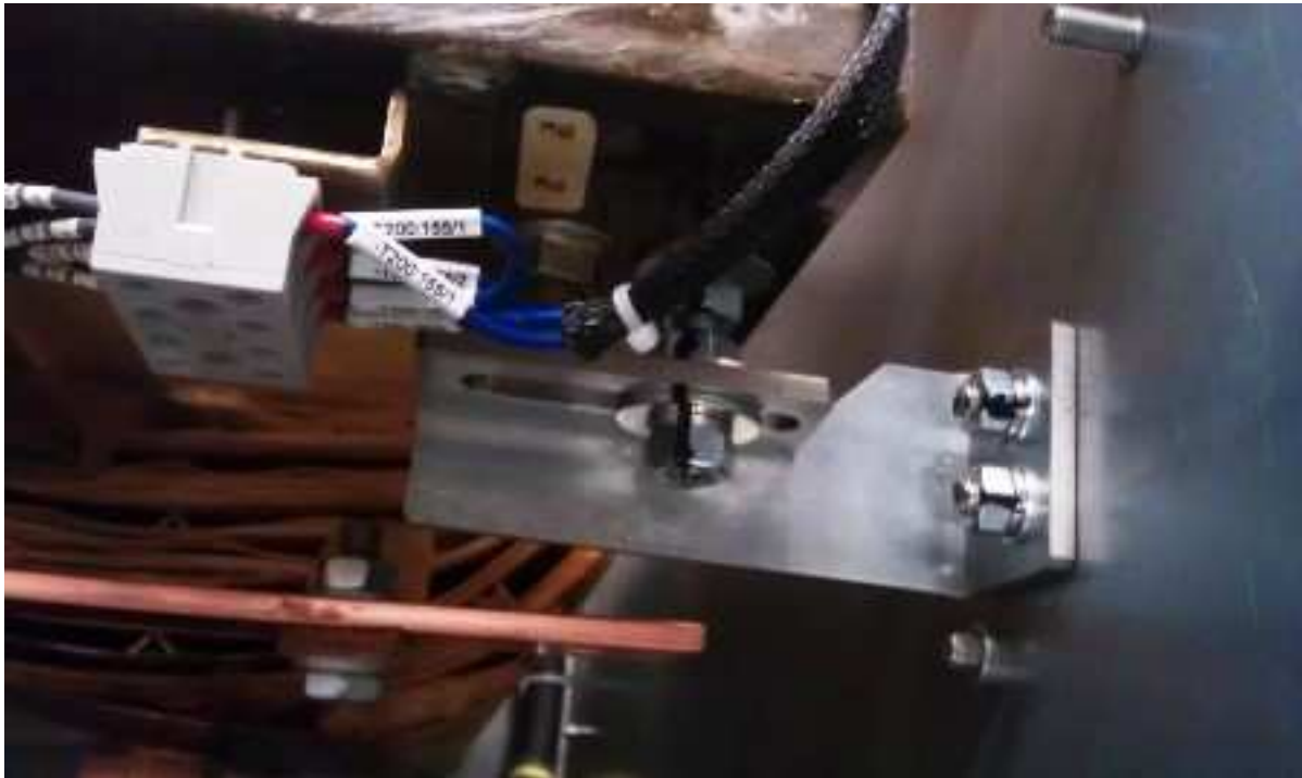
Figure 6-4 Transformer fixing on the right side
