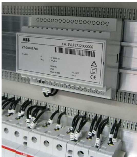
Fig. 5 – VT Guard Pro, placed in LV switchgear compartment
