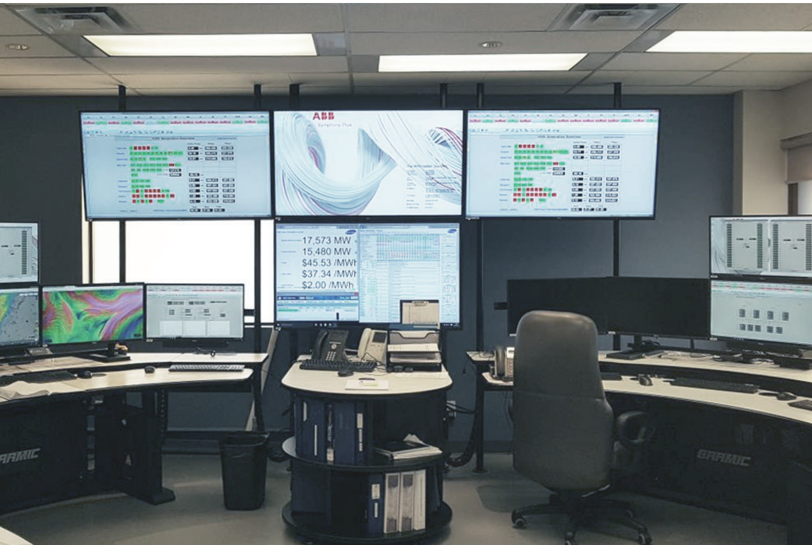
20 The new H2O Power control center in Ontario enables a single operator to manage 48 units efficiently and safely
