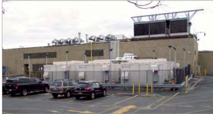
Figure A1-1 – Seven 200 kW fuel cells at Verizon's Garden City Central Office on 3 rd November 2012 [23]
