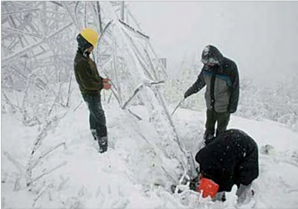
Figure A3 – Ice-damaged transmission tower, China [1]
