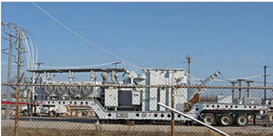
Figure A4-4 – Portable transformer used to restore service in a damaged substation [24]
