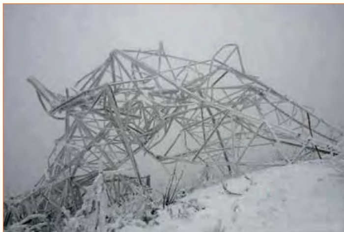
Figure 2-1 – Ice damage to power line in China, 2008 [1]
