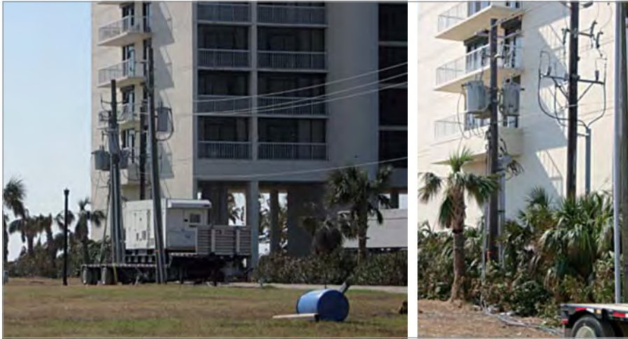
Figure A4-3 – Apartment complex in Galveston Island, Texas, powered by a portable generator connected to the distribution portion of the grid [24]
