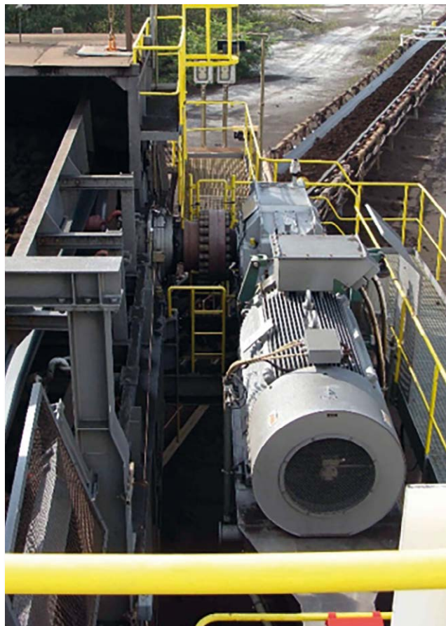
Figure 2: View of a typical belt conveyor drive with gearbox
