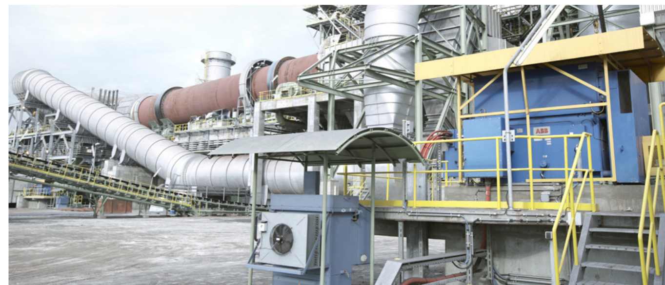
Figure 1 Flowmeters typically sited in harsh environment
