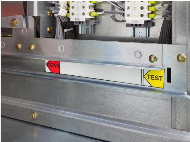
Figure 4.23 Circuit breaker position indicator
