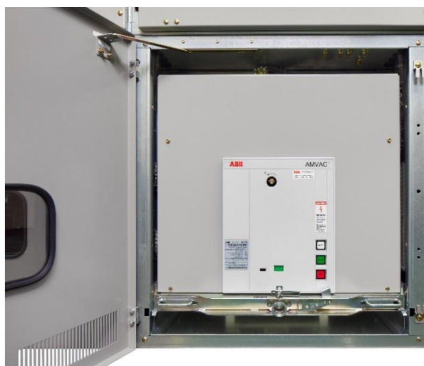
Figure 4.21 Circuit breaker in DISCONNECT position
