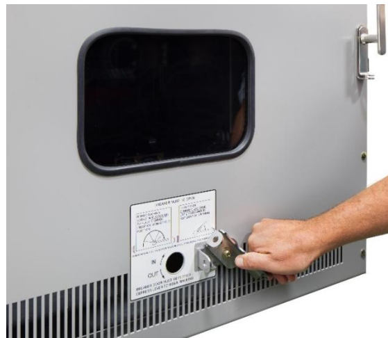
Figure 4.22 Racking release handle
