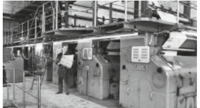
In the mid-1960s, prior to the introduction of modern variable speed drives, ABB's forerunner delivered drive and control systems for the printing presses at Sweden's largest newspapers, including Svenska Dagbladet, shown here.
