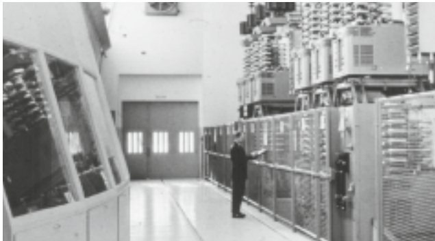
A technician in the Gotland valve hall, part of the world's first commercial HVDC transmission system, commissioned in 1954.
