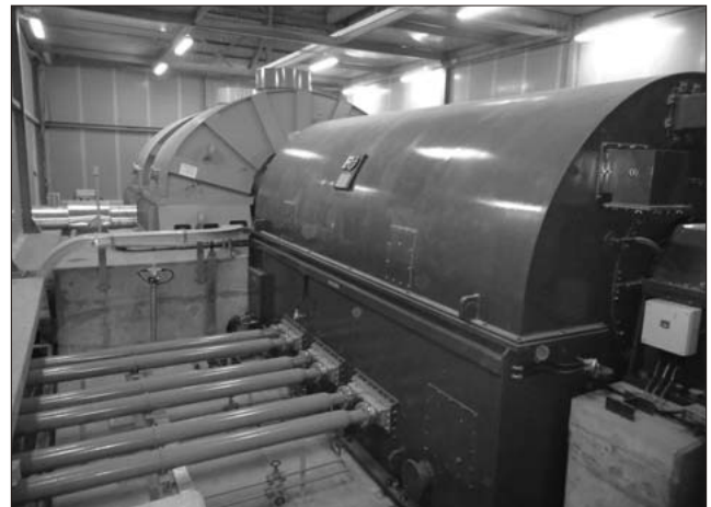
Fig.10 Turbine and generator of Unit 3 of Ulubelu Geothermal Power Plant
