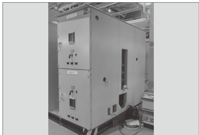
Fig.5 High-voltage switchboard for seismic resistance verification
