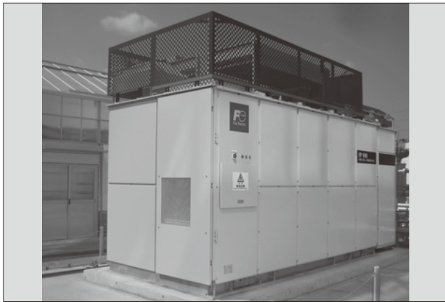
Fig.3 Fuel cell facilities installed in Tokyo Factory
