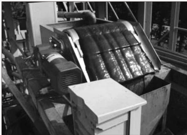
Fig.10 Sludge-less wastewater treatment system (magnetic separator)
