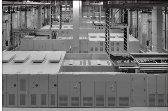
Fig.2 Installation status of power conditioning equipment
