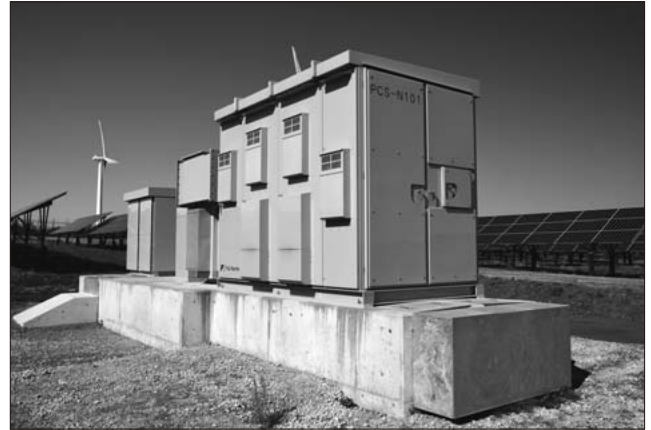
Fig.4 Installation state of PCS, booster transformer and ring main unit
