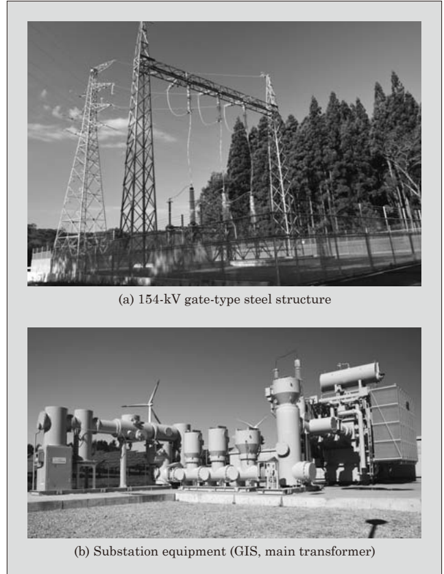
Fig.5 154-kV gate-type steel structure and substation
