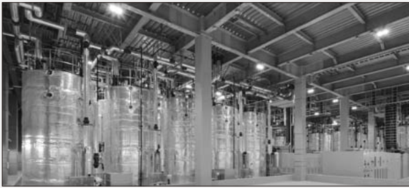
Fig.7 Large electric power storage system of Minami-Hayakita Substation
