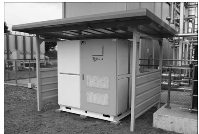
Fig.10 Steam generation heat pump under field testing
