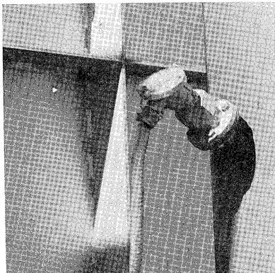
Fig. 5 Detecting element for temperature of raw material in preheater
