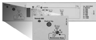
Close-Up of LG Trip Unit
